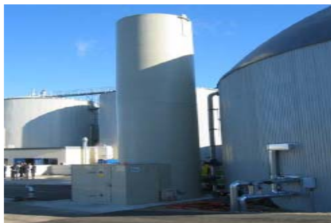
digester, biogas desulphurisation and post digester
