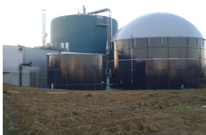
digester and post digester
