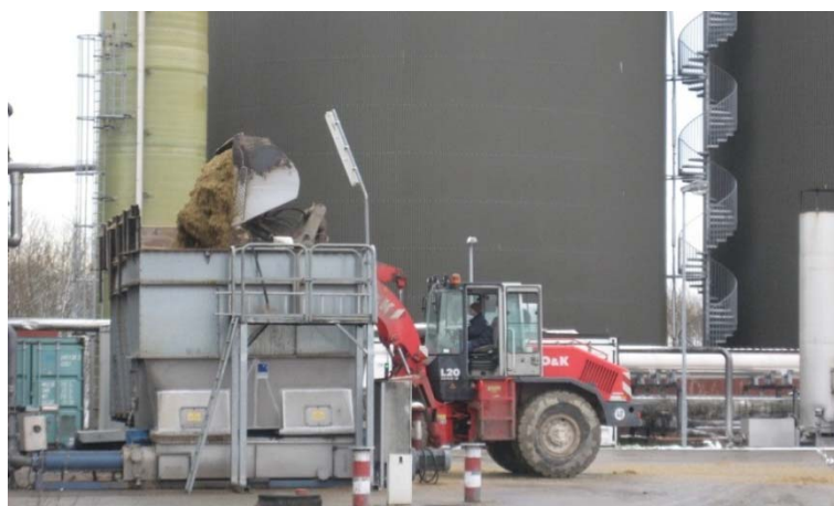
reception tank and digesters
