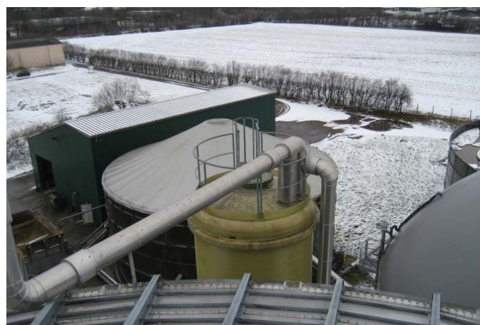
hydrolysis, desulphurisation, post digester
