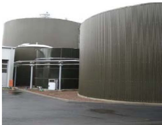
digester and waste water treatment plant
