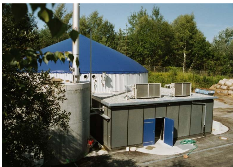
digester, machine hall
