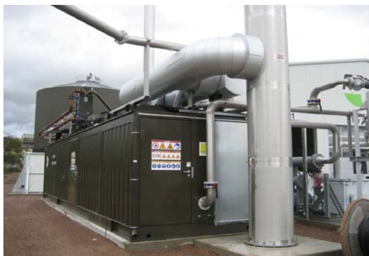
digester and co-generation plant
