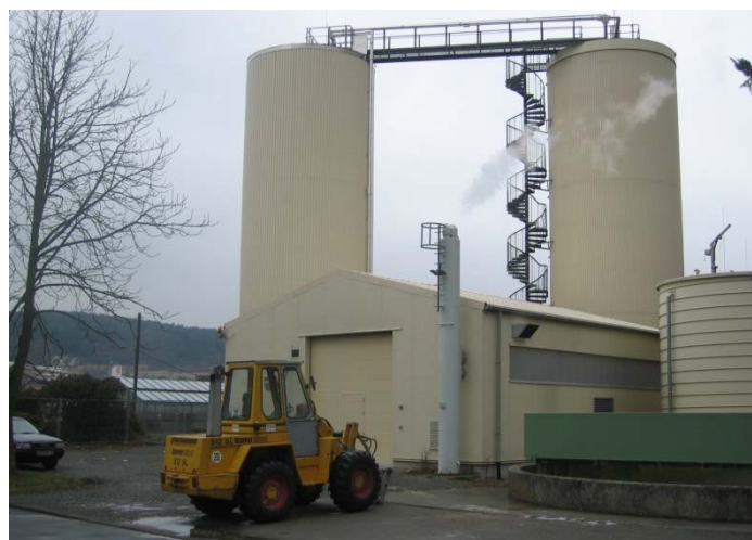
high performance digester
