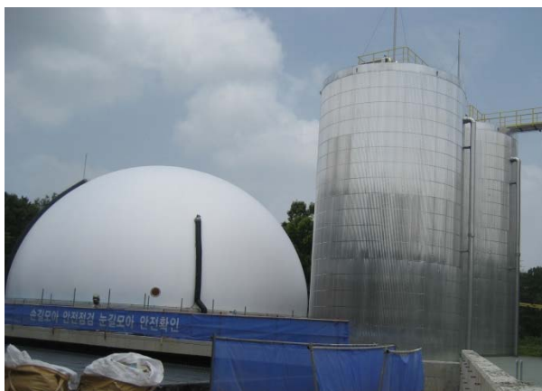
digesters, digestate storage, machine hall
