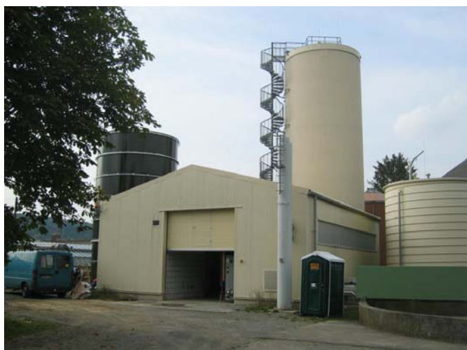
high performance digester
