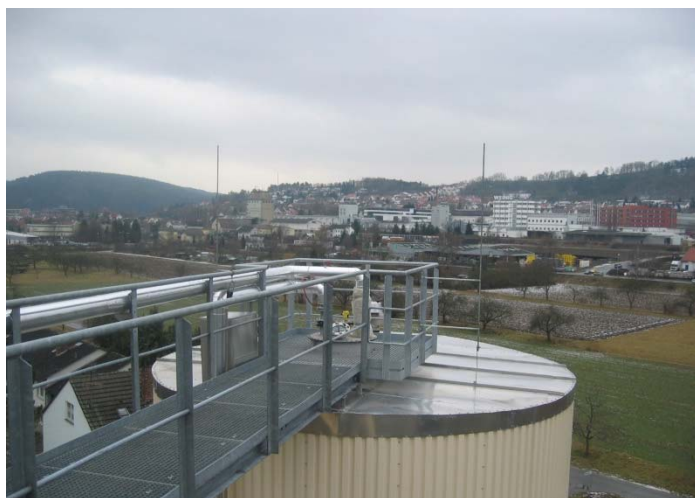
roof of high performance digester
