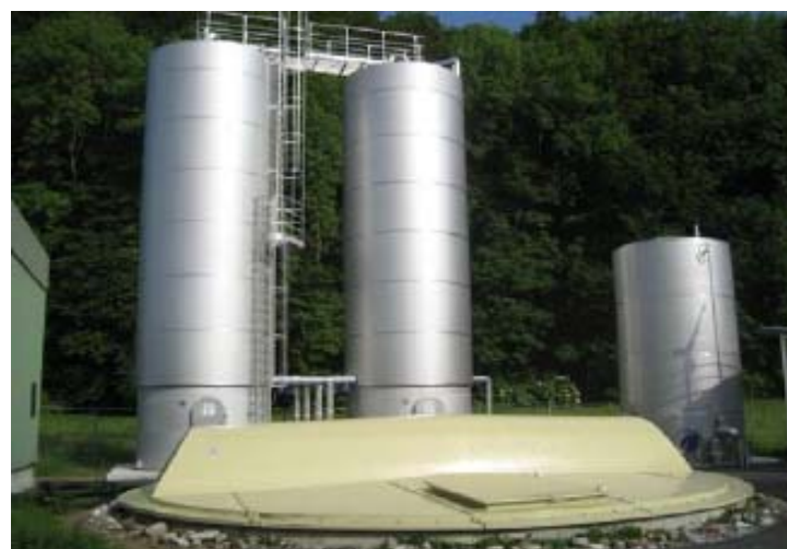
high performance digesters
