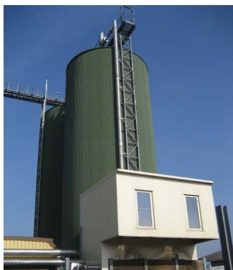
high performance digester
