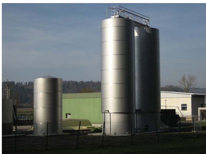
high performance digesters
